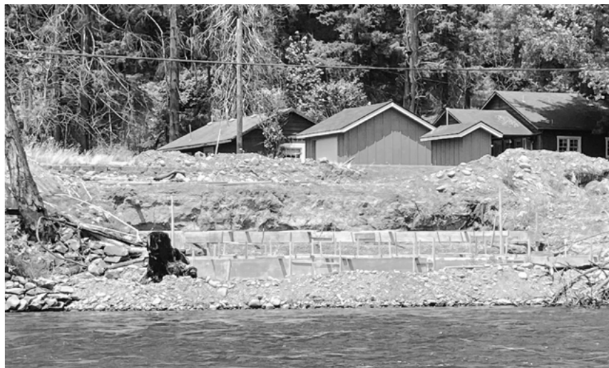
Excavation, house foundation and removal of all vegetation in the riparian zone
