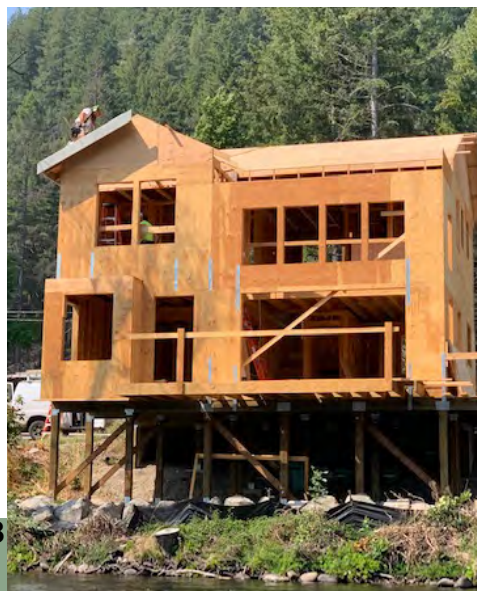
Right and below, houses permitted by HB 2289 in direct violation of Lane County's riparian ordinance and the requirements of the Division of State Lands
