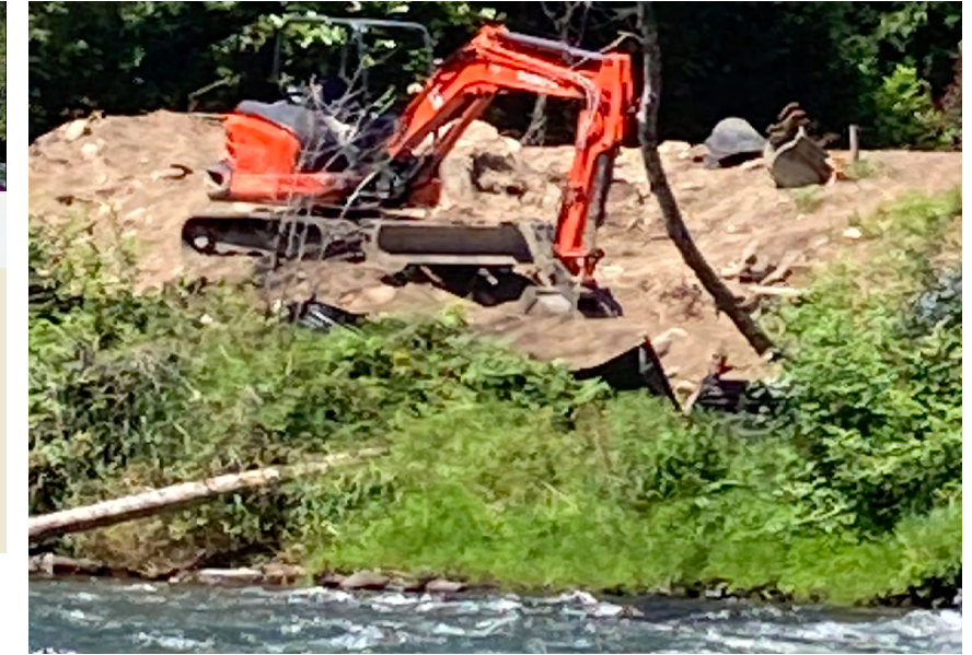
An excavator at work disturbing precious riverine soils near the water's edge
